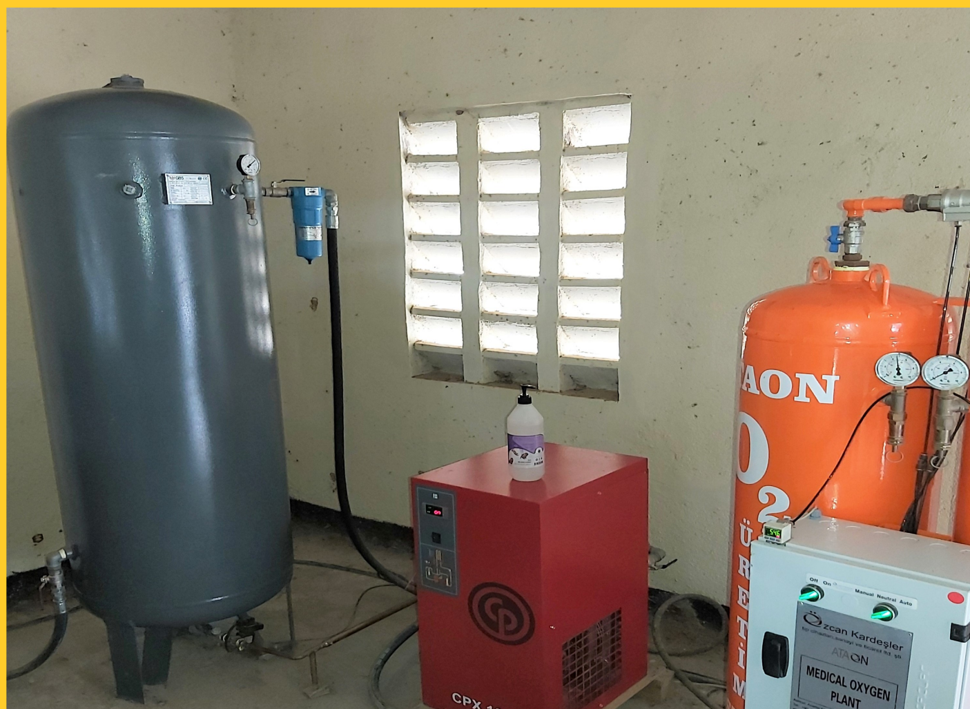
Medical Oxygen Plant Installed at Garba tulla Level IV Hospital in Isiolo County
