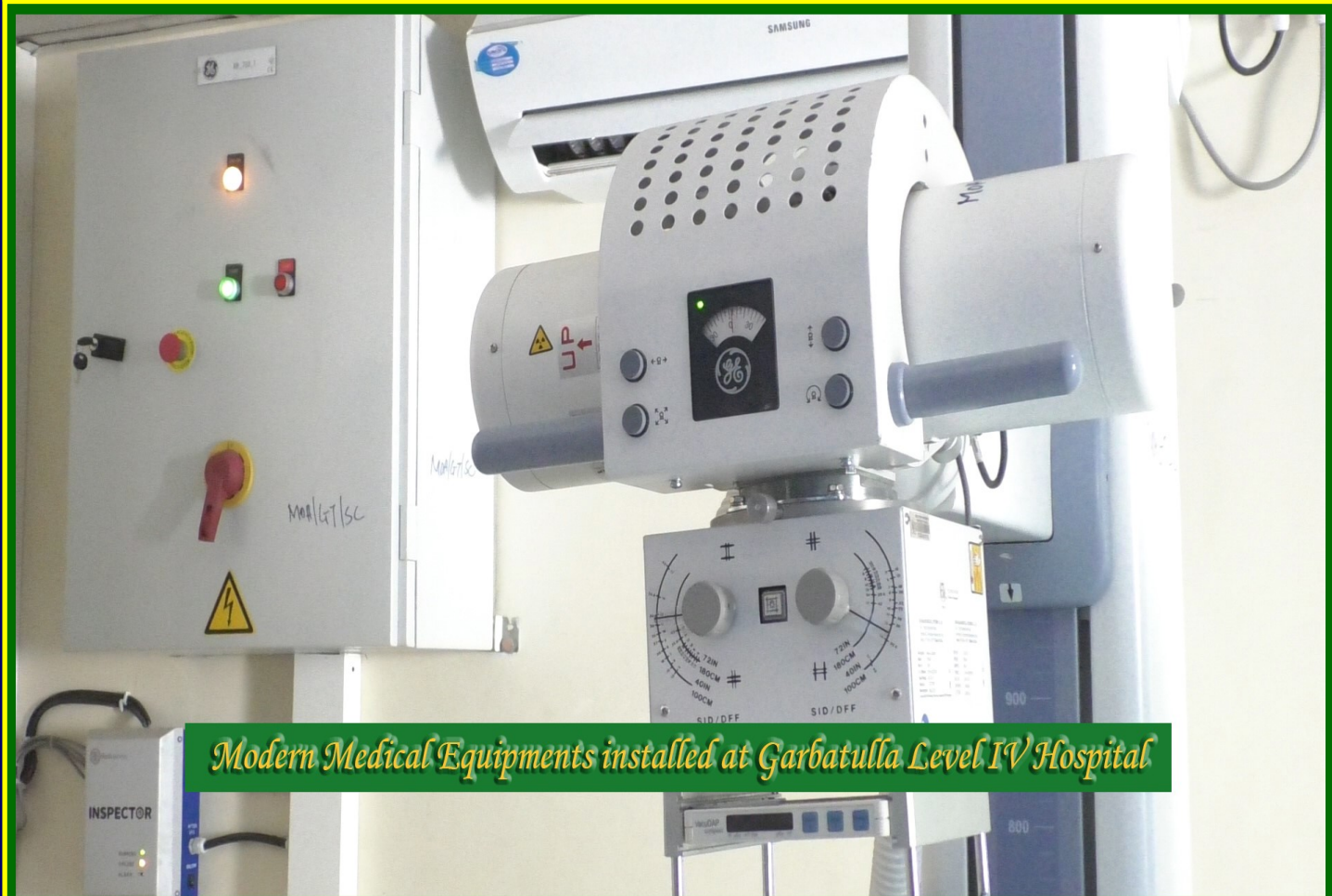
Modern Medical Equipments installed at Garbatulla Level IV Hospital
