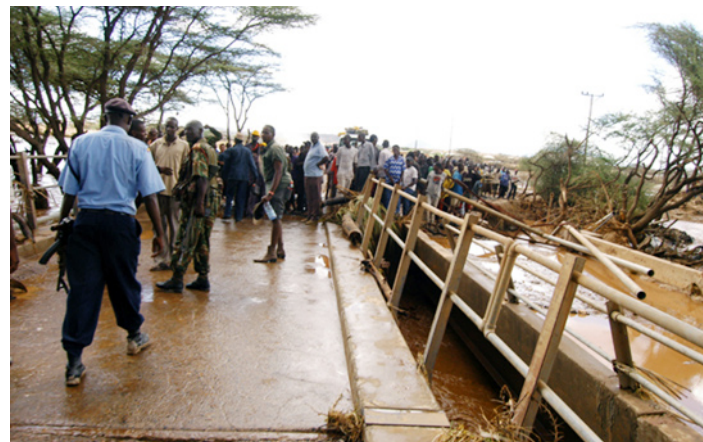
Plate 7.1: A bridge over the Ewaso Nyiro River at Archers Post damaged by flood waters (Source: Daily Nation)
